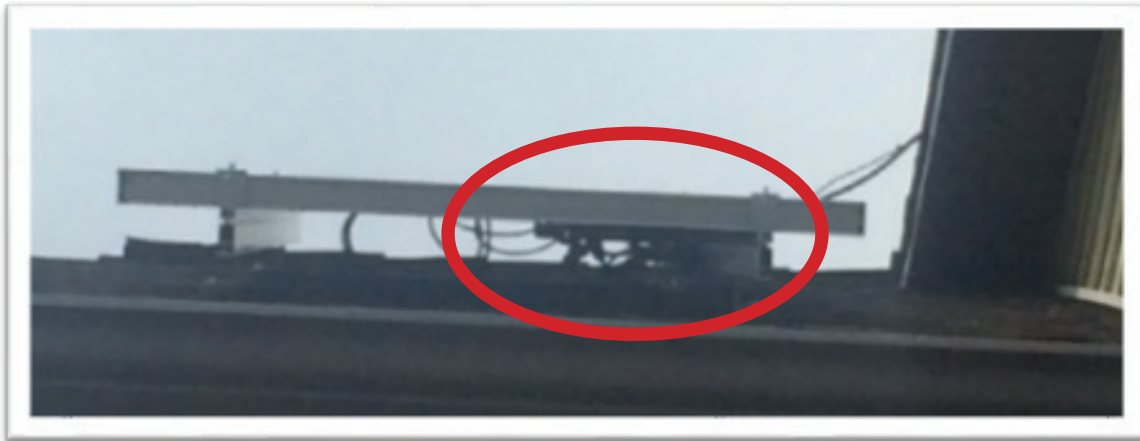
Photo D8: Source circuit conductors in contact with roof: NEC 338.10
