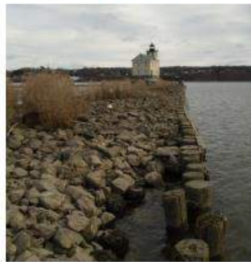
Erosion along the jetty, observed in January 2019
