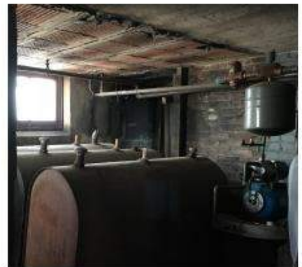
The lighthouse basement, which lacks utility connections
