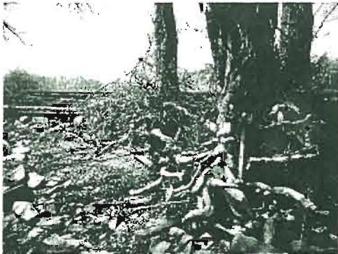
Figure 4 – Exposed tree roots along Kingston Point Causeway
