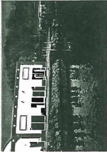
Figure 15 - Scour and undermined pavement.
